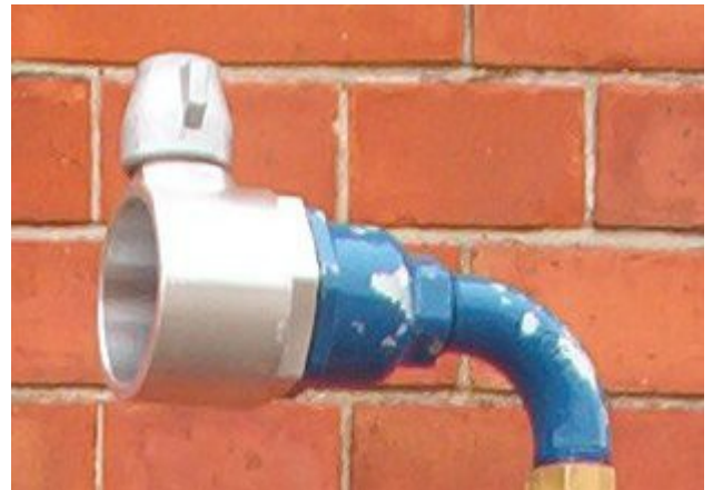
Fire hose connection
